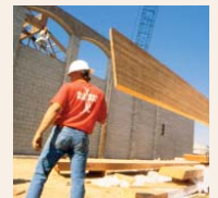
Massive glulam timbers, spanning 115 feet, are being installed here to provide structure & decorative framing for the Unified Physical Education & Sports Complex in Coronado, CA. SHWC Architects reported, "steel could not have provided the dramatic design focus achieved with the exposed laminated trusses."
